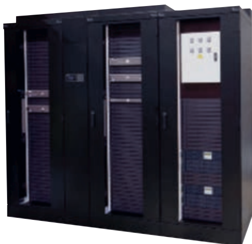
Solution de micro data center
